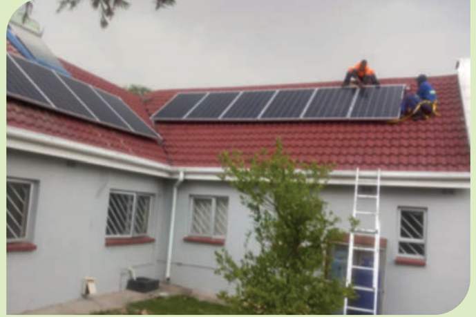
5kw Solar system residential installation
