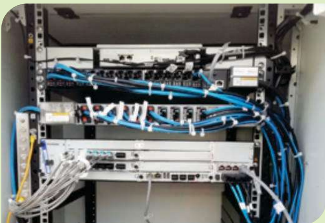
Huawei installation 5G network
