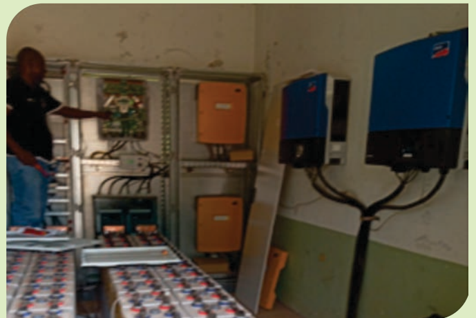
Solar For Health 40KW grid-tied installation with 18kwh storage
