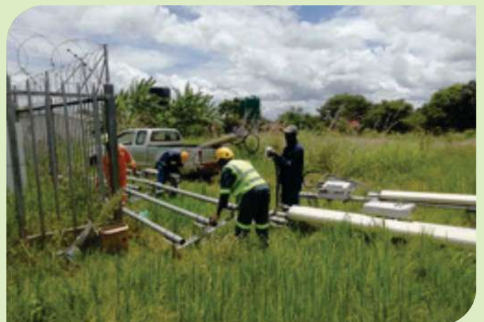
4G Ericson Installation
